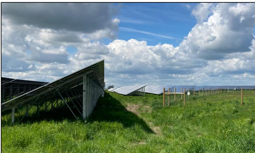
Plate 3.2 Example of a typical mounting structure
